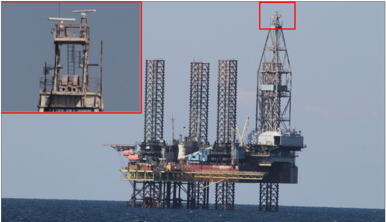
Photo 4. The NEVA-type radars installed on the TAVRIDA Jack-up Drilling Rig, captured as part of the Ukrainian state company Chornomornaftogaz on the Odeske gas field.
