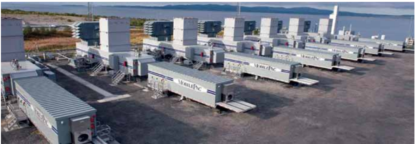
Picture 1, 2. Mobile GTPP Gas Turbine MOBILEPAC Package, produced of the American PW Power Systems LLC.
